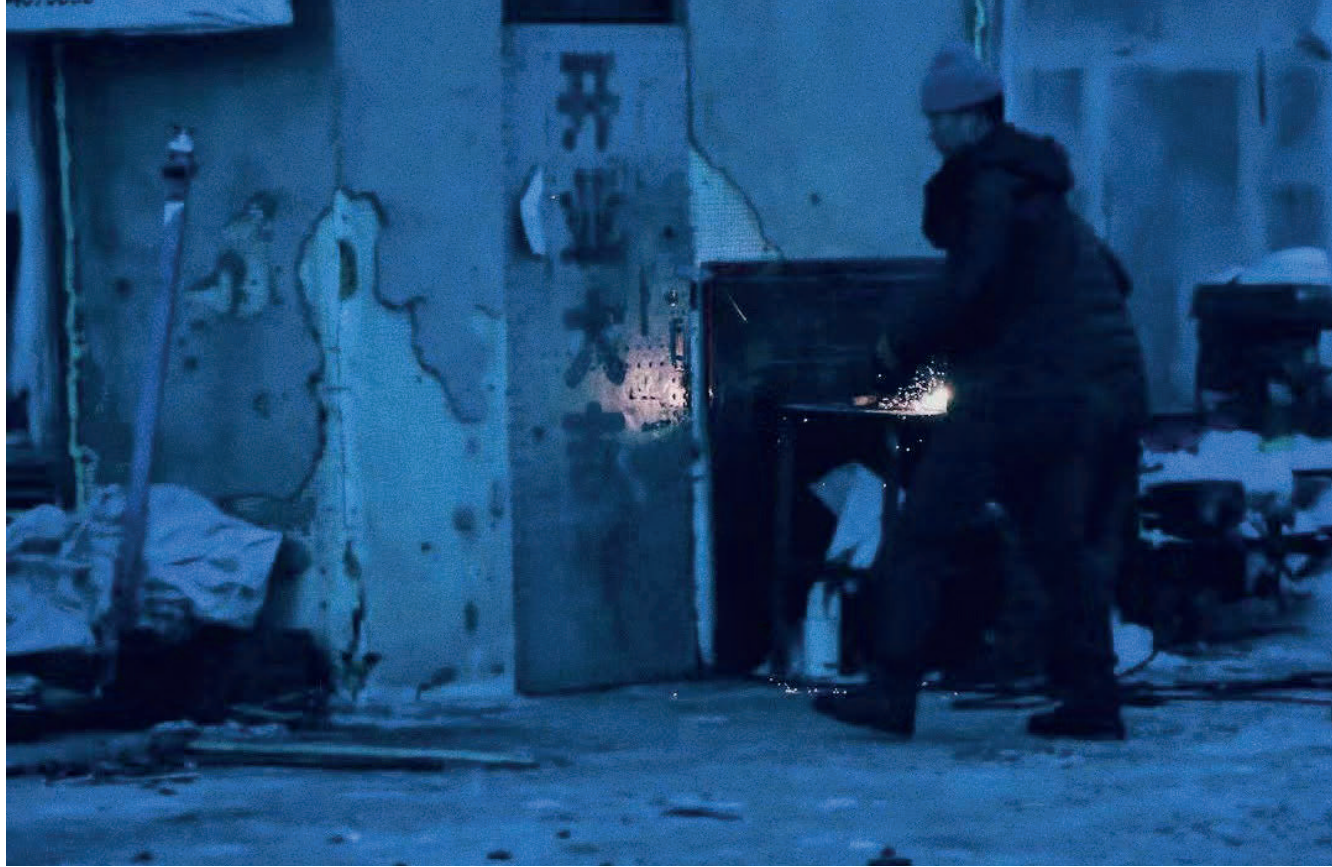
Evening in Beiji Village. from the travel log of Hui, 2020. A worker welding.
