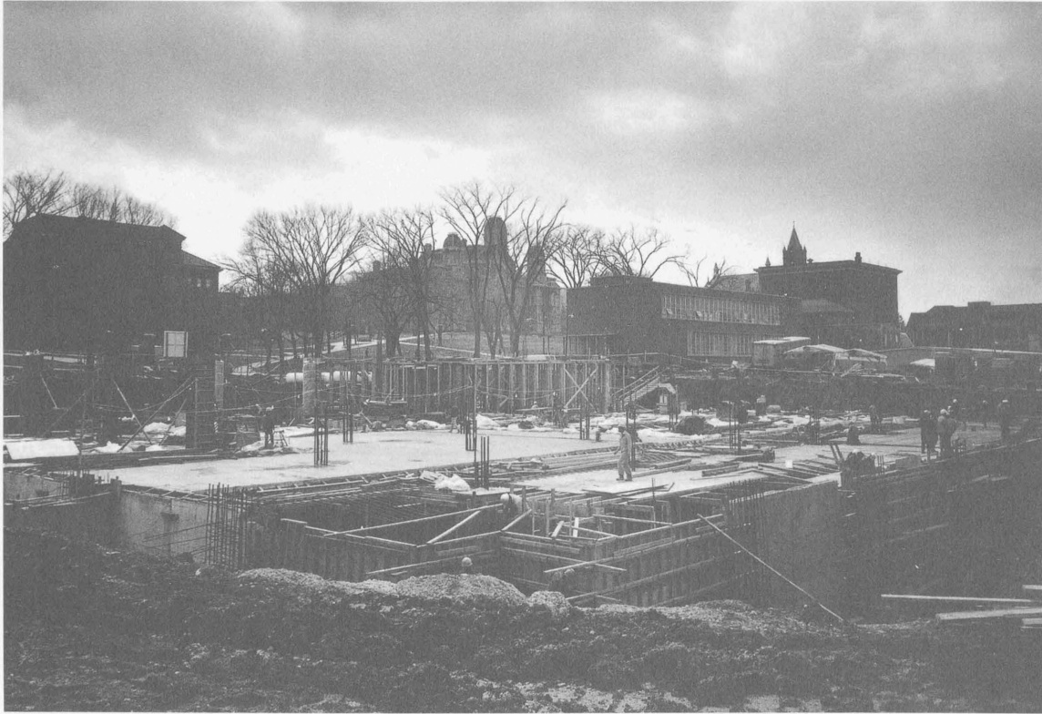
Construction of E. S. Bird Library, 1970 (This and the following photo are courtesy of Syracuse University Archives).
