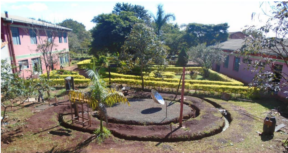
Image 8. Beginning of the Grey Water Filtration System being built between the Refectory (left) and Main Office Building (right). A sun oven is pictured in the center of the system. Photo by author.
