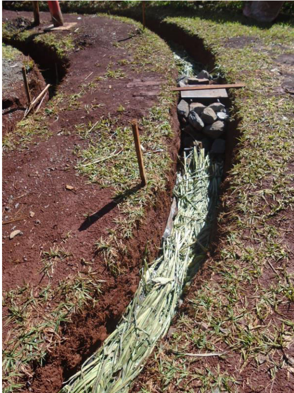
Image 9. Water sampling chamber along the trench. Photo by author.
