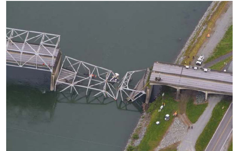
Fig 3.1 I-5 Skagit River Bridge collapse
