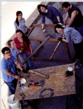
Students work on floor boards that have been ripped up and will be recycled into the 601 Tully project
