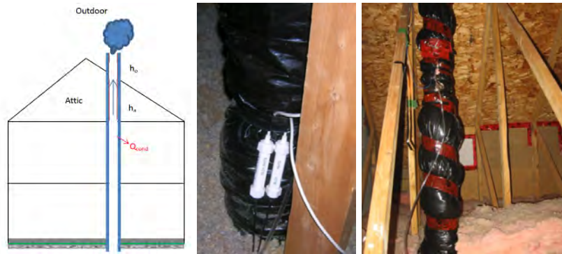
Figure 1. The schematic of system modeled (Left), Temperature sensor in the stack in the attic (Middle), and insulation around the stack in the attic (right).
