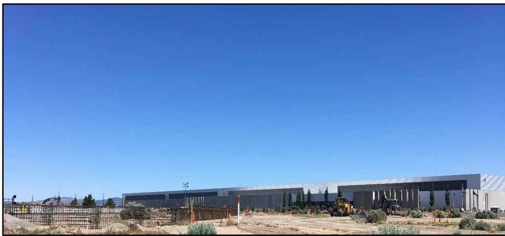
Figure 3. A view of the Facebook data center from Tom McCall Road in Prineville, Oregon. The bulldozers located around the site are a constant presence. Plans for construction of a fourth data center are currently underway. Photo by author.
