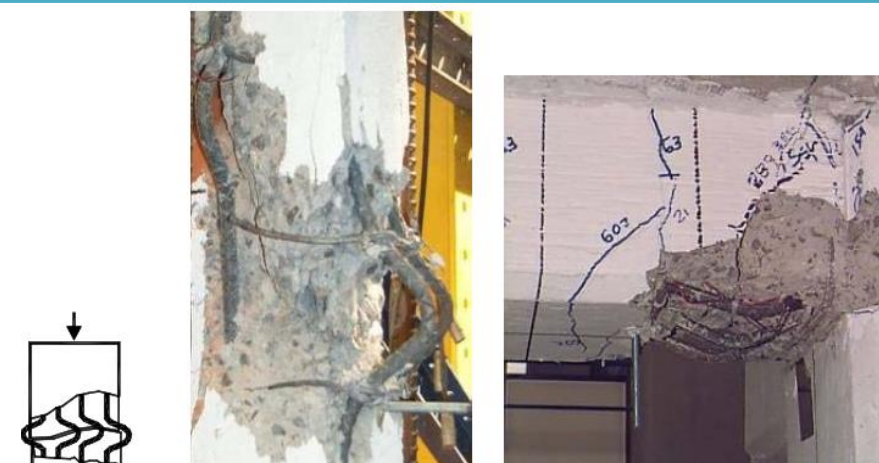
Figure 3. Damage in concrete elements (CENAPRED, 2011)
