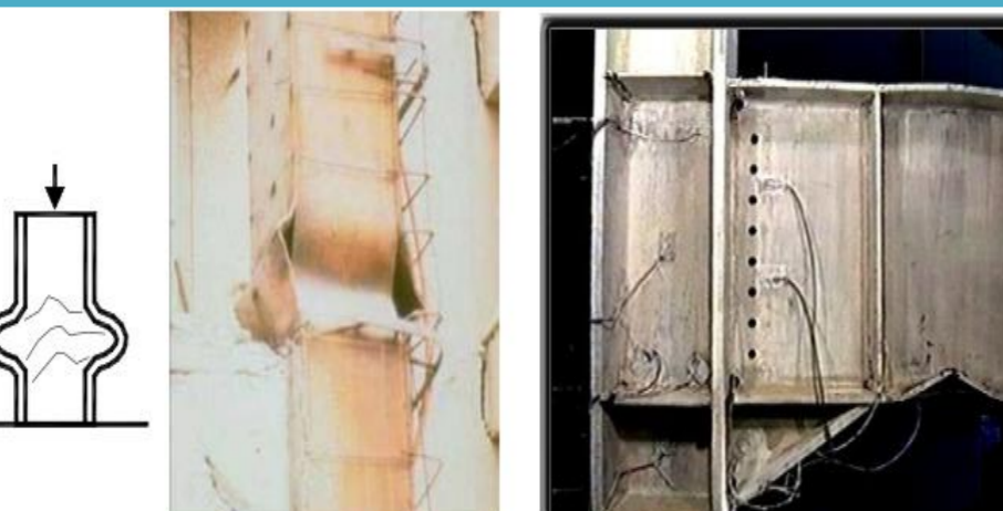
Figure 4. Damage in steel elements (CENAPRED, 2011)
