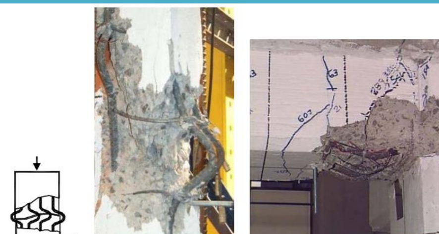
Figure 3. Damage in concrete elements (CENAPRED, 2011)
