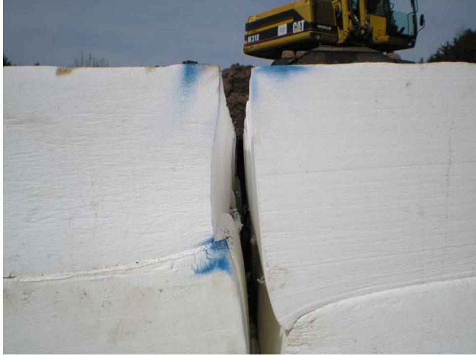
Figure 2.14 Geofoam joints and differential settlement at Carrs Creek (NYSDOT, 2007)
