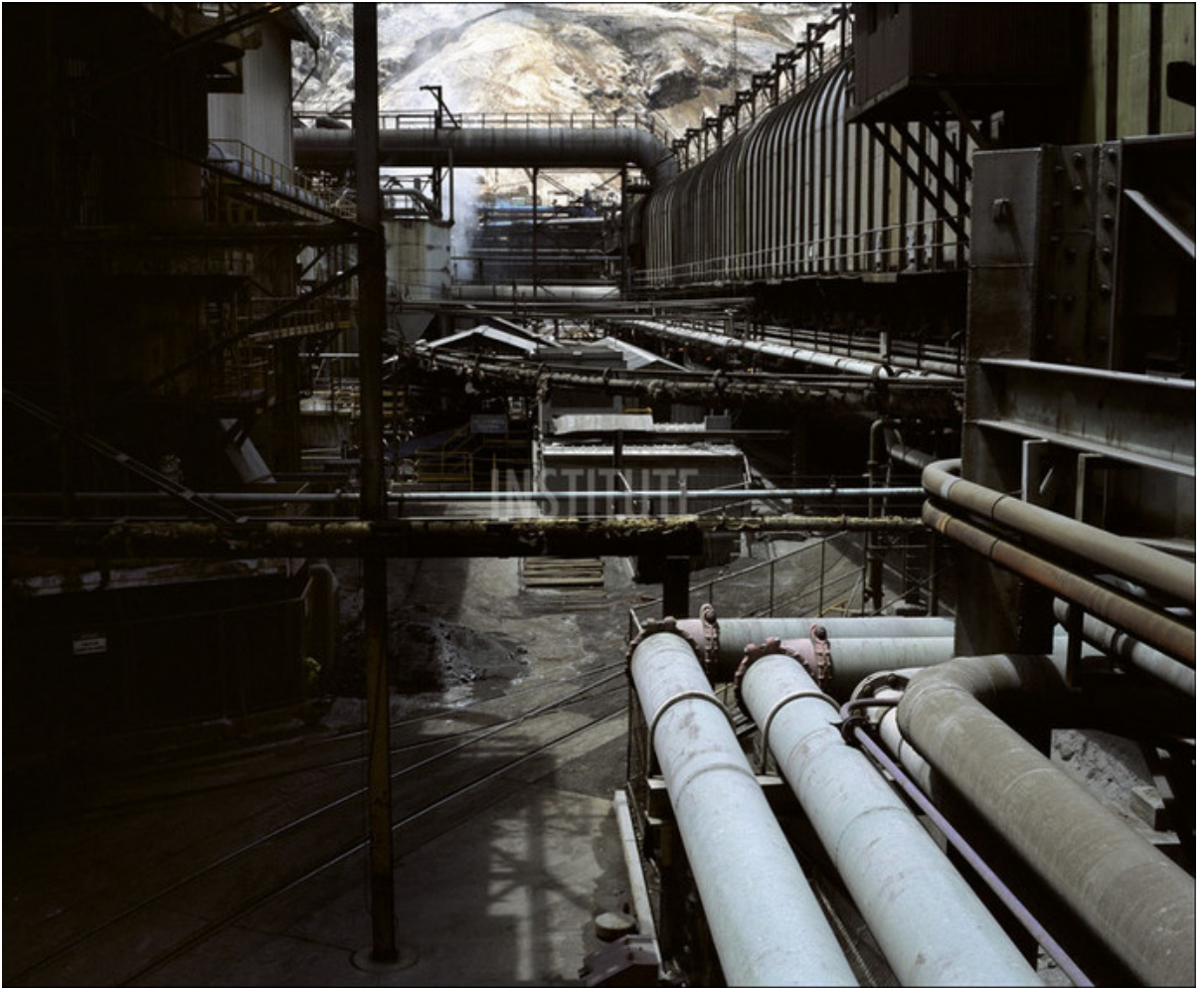
Water importation and filtration facility. Germany.
