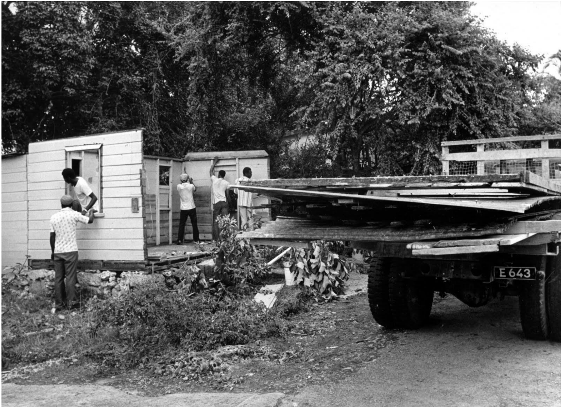
Figure 5.1: Community residents disassembling a chattel house in the parish of St. Peter. Photo from http://islandman48.blogspot.com/2009/11/there-is-little-that-tells-as-much.html
