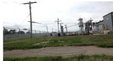
Figure 3: Downed conductor on a High Impedance Surface [2]
