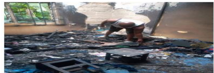
Figure 2: Scene of a recent fire incident in Nigeria caused by HIF
