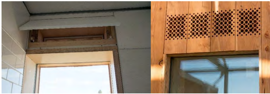
Figure 3: Ventilator as seen from inside test house (left).
