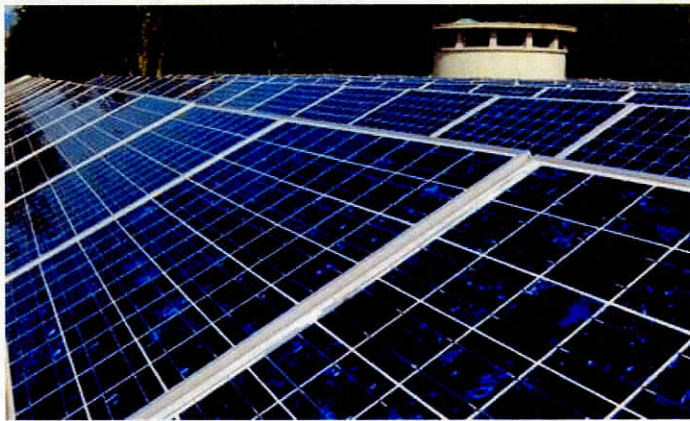
Rows of Photovoltaic arrays
