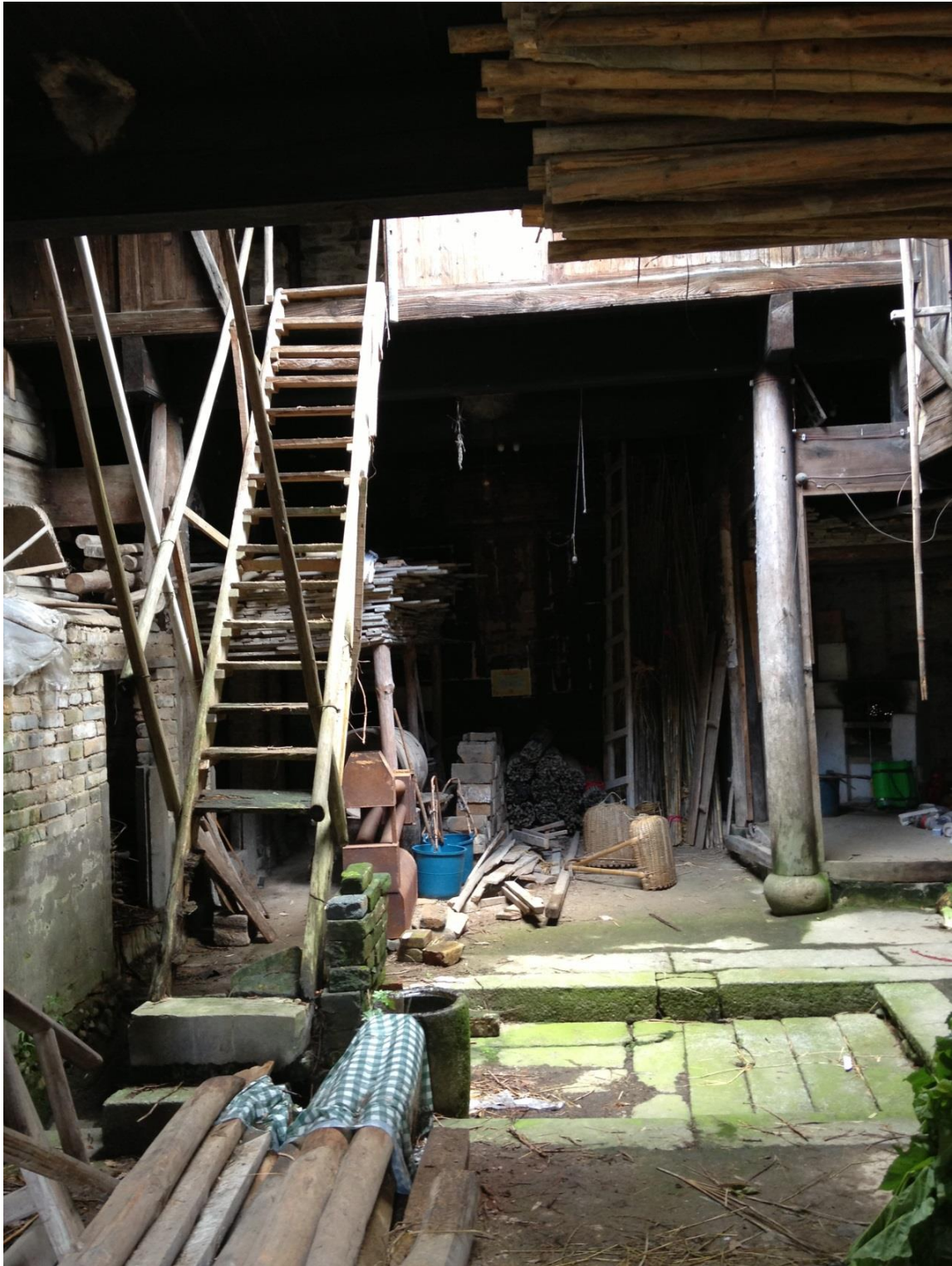
Figure 5.8: Dilapidated historical house in Xucun. (By author.)
