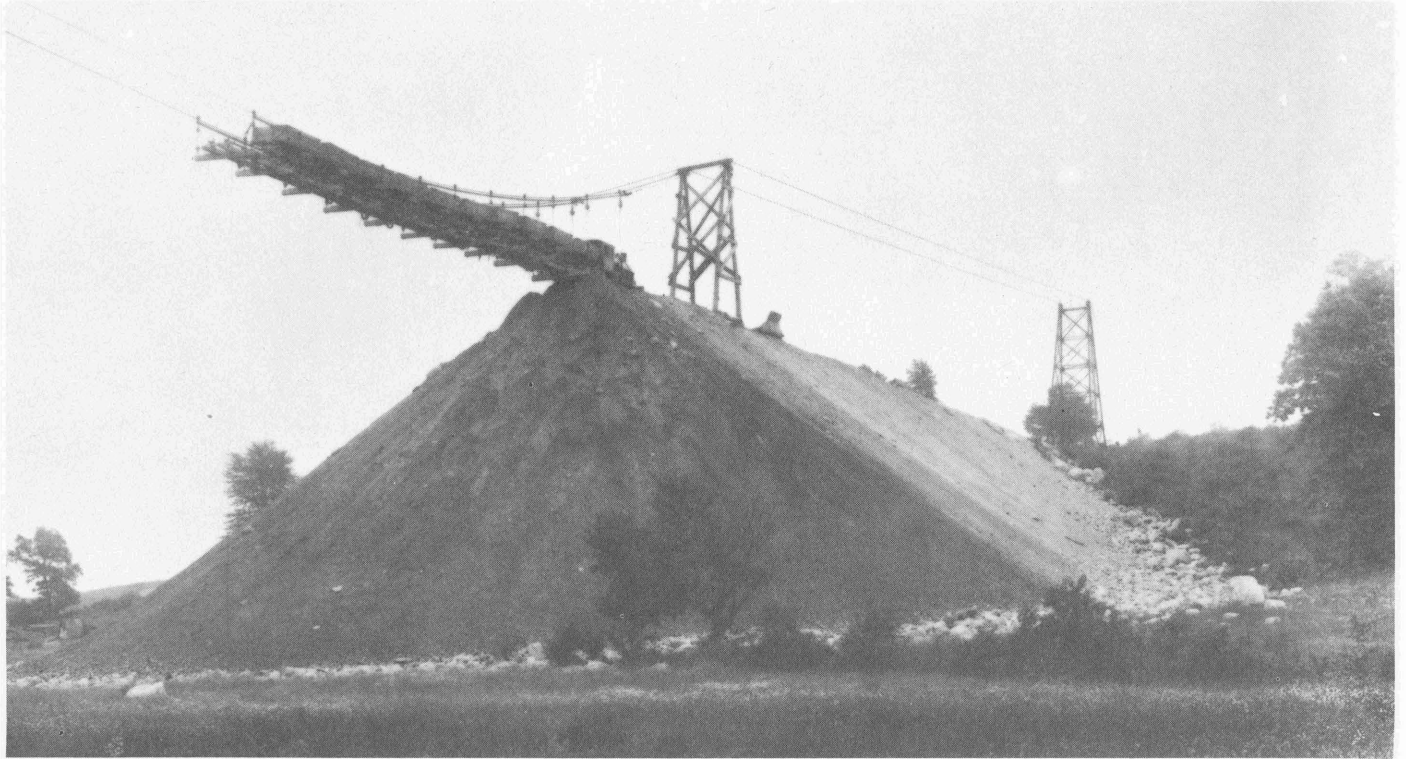
Cable-suspended track from which dump-car trains dropped fill material to create an embankment for a new railroad line. July 7, 1910
