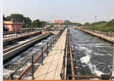
16.5 MGD treatment capacity Waste water treatment plant in Jaipur.
