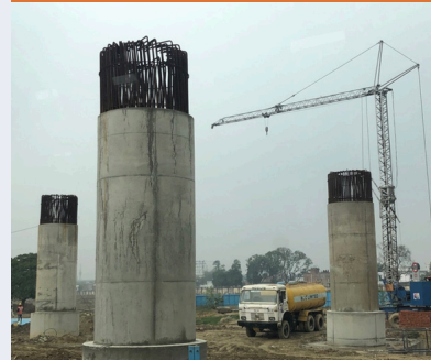
Using India's own construction equipment for the remodeling of Lucknow international airport
